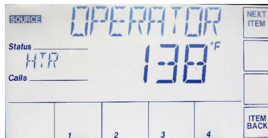
Figure 10-8 Setting the Setpoint
