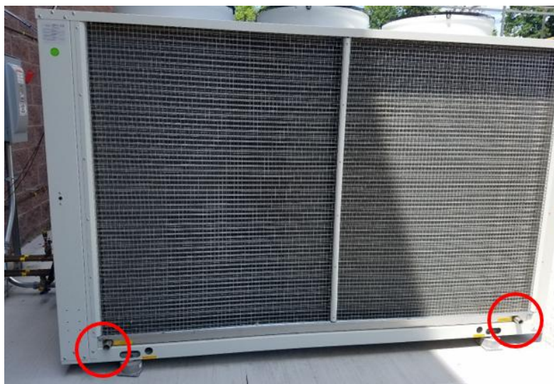
Condensate Drain Pipes
