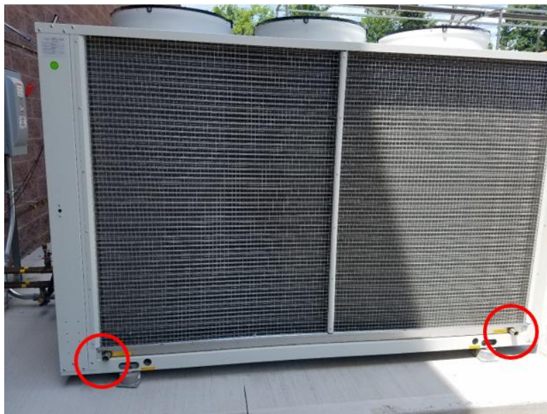
Condensate Drain Pipes
